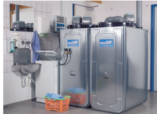
Plant type MF-HKA4, installed in a cellar
